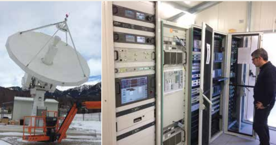
An MTG telemetry tracking and control ground station and its shelter in Cheia, Romania
