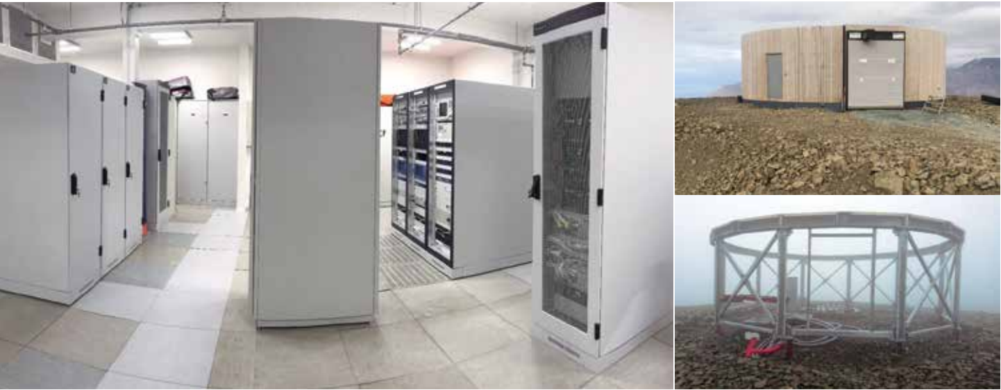
Hosting infrastructure for Ka-band antenna (top right) and S-band antenna (bottom right) and command and control shelter (left) at Svalbard
