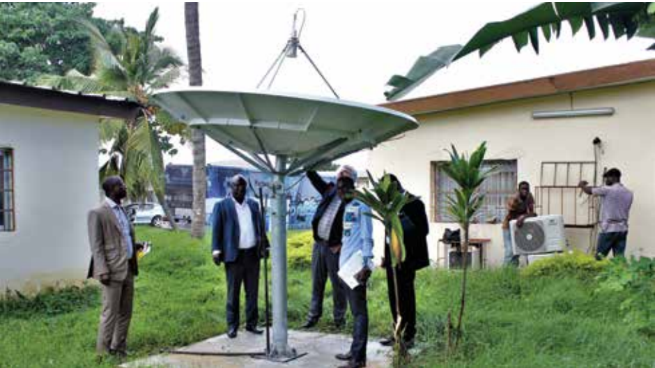
Setup of a new antenna in Abidjan as part of the migration to the new EUMETCast-Africa service, implementing the DVB-S2 standard
