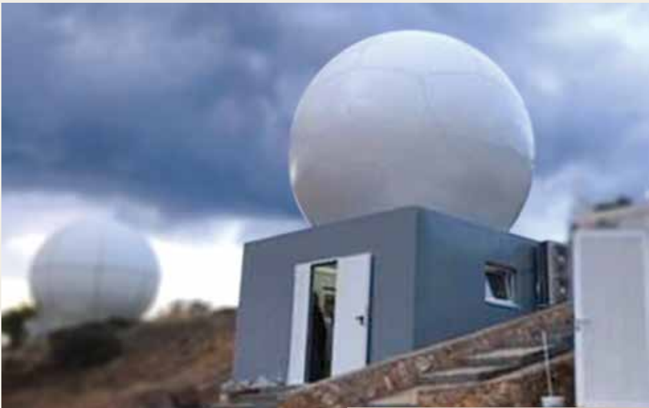
The Athens EUMETSAT Advanced Retransmission Service (EARS) station is now equipped with two X/L-band antennas
